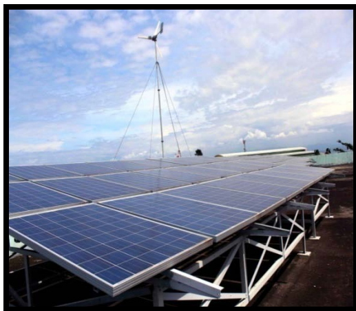
Figure 4. PV Arrays and wind turbine
