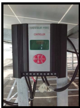
Figure 5. Wind and Solar Hybrid Controller
