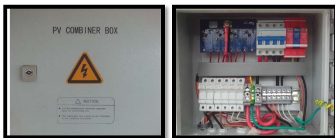
Figure 6. PV Combiner Box
