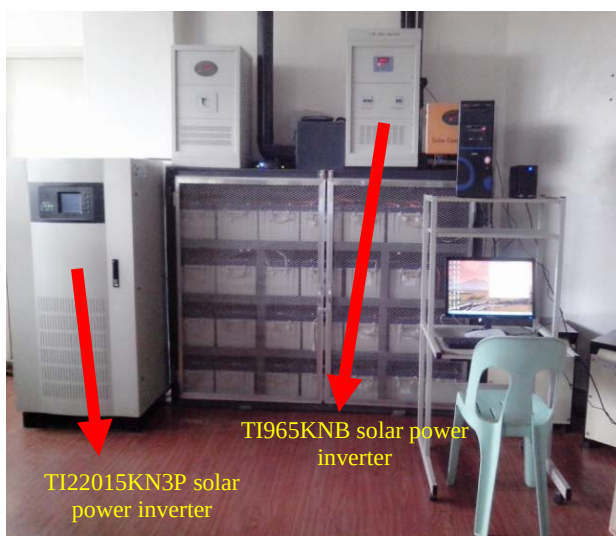
Figure 9. Charge controller, inverters, batteries and monitoring system
