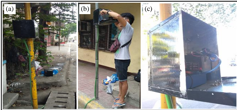
Figure 6. Actual system deployment at M.J. Cuenco Avenue (a), Eduardo Aboitiz Street (b), and Bonifacio Street (c)
