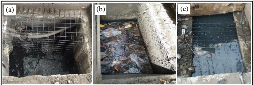
Figure 3. The actual drainage status of the manhole in M.J. Cuenco Avenue (a), Eduardo Aboitiz Street (b), and Bonifacio Street (c) before actual system deployment
