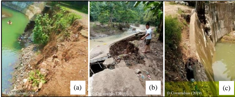
Figure 1. Slope protection structure failures in Zamboanga City, Philippines on September 13, 2019 – Sinunuc River (a), Lunzurun River (b), and Divisoria-Putik River (c)
